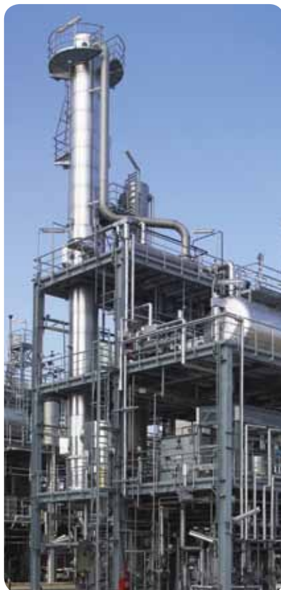
Chemical processing plants
